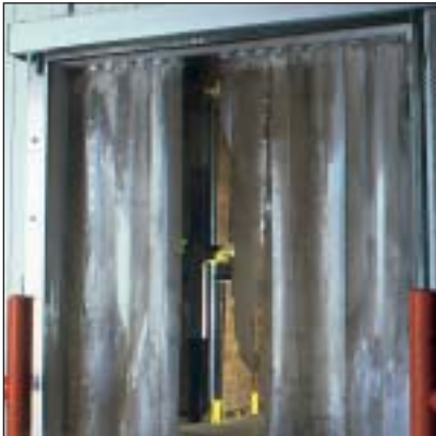
Broken plastic strips do not screen off the doorway properly.
